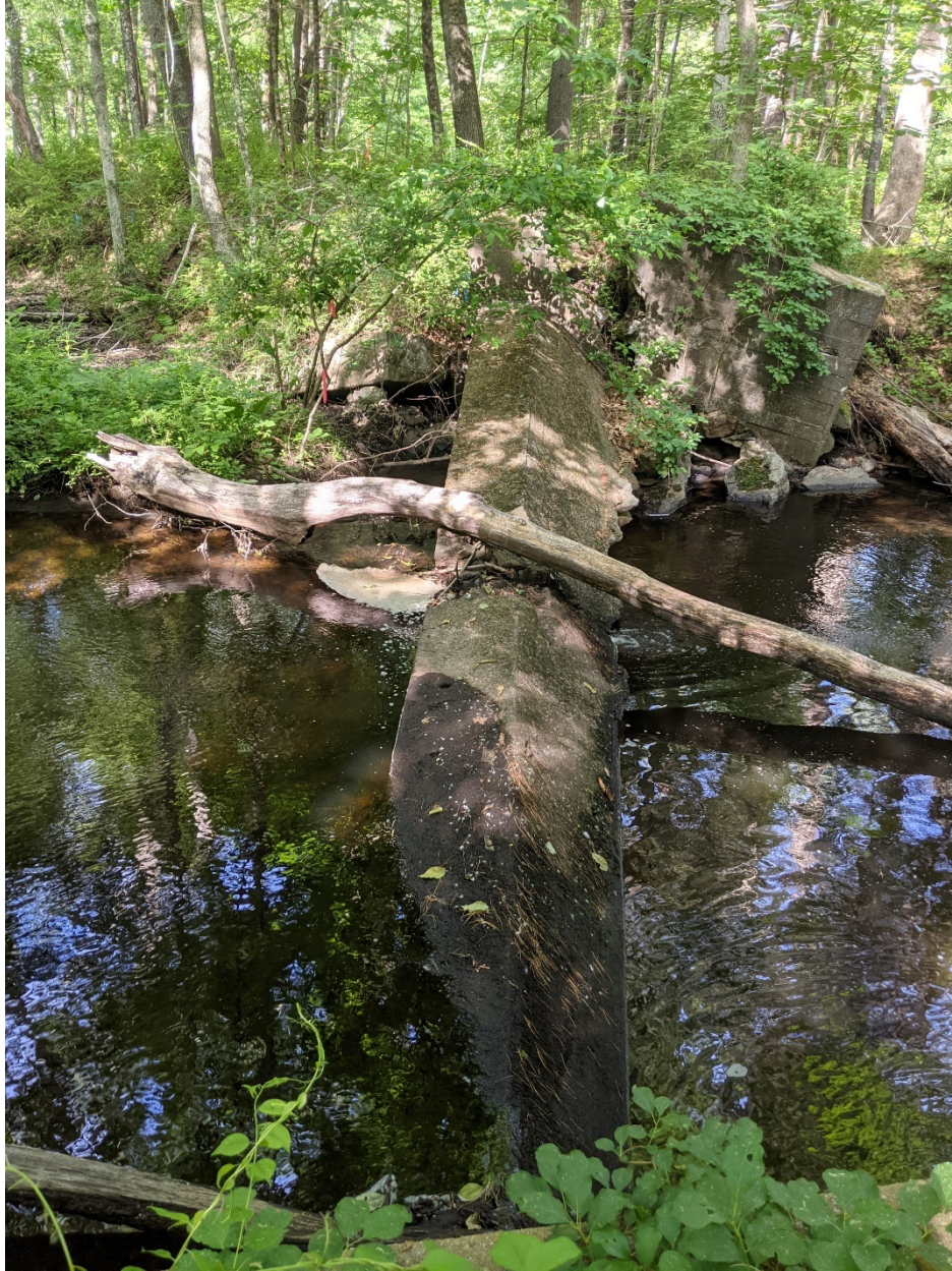
Photo 4: Collapsed spillway. Note that very little water flows over the collapsed spillway currently, as most flow goes underneath the undermined portion.
