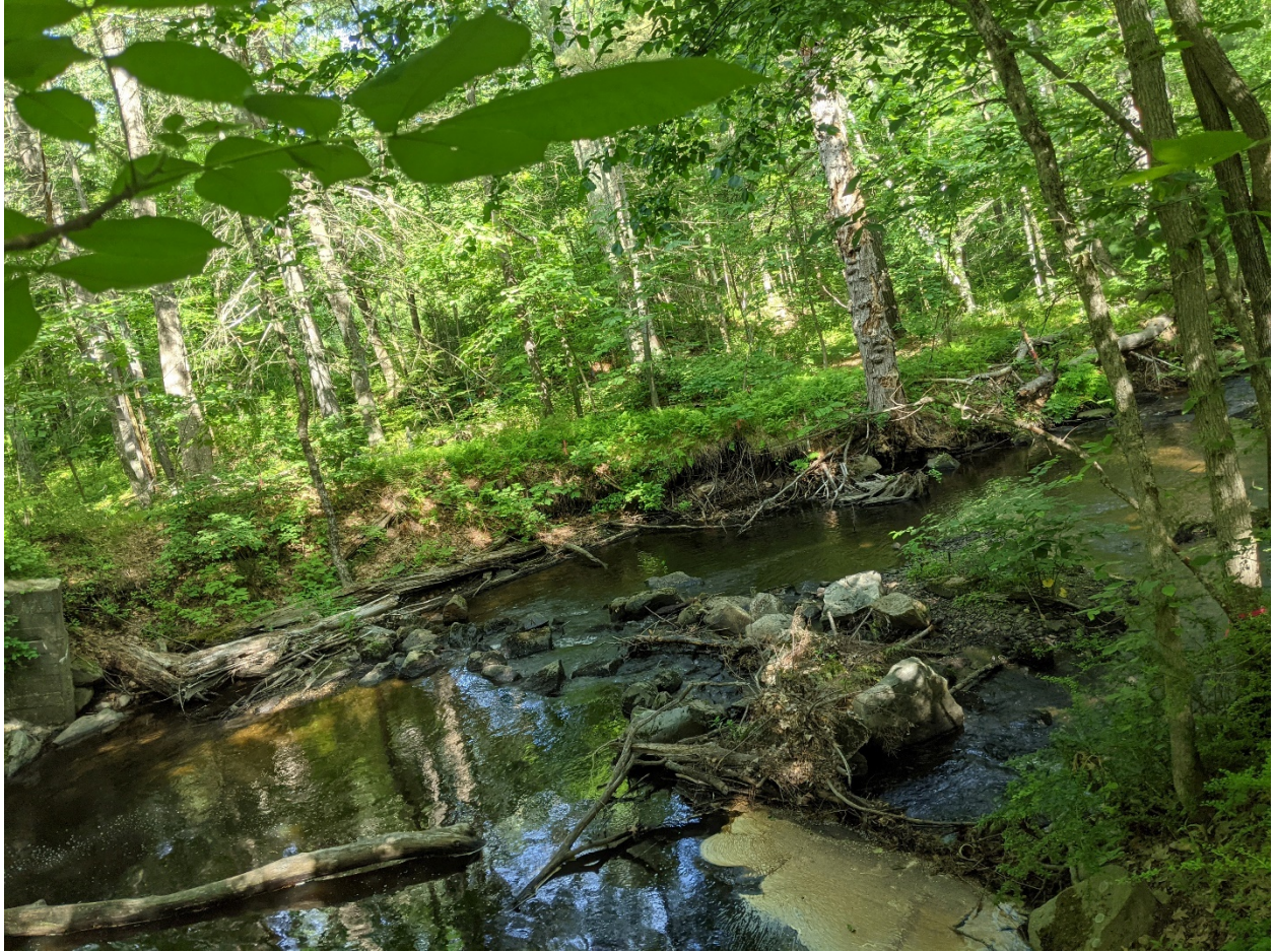
Photo 2: Rock riffle immediately downstream of the collapsed spillway.
