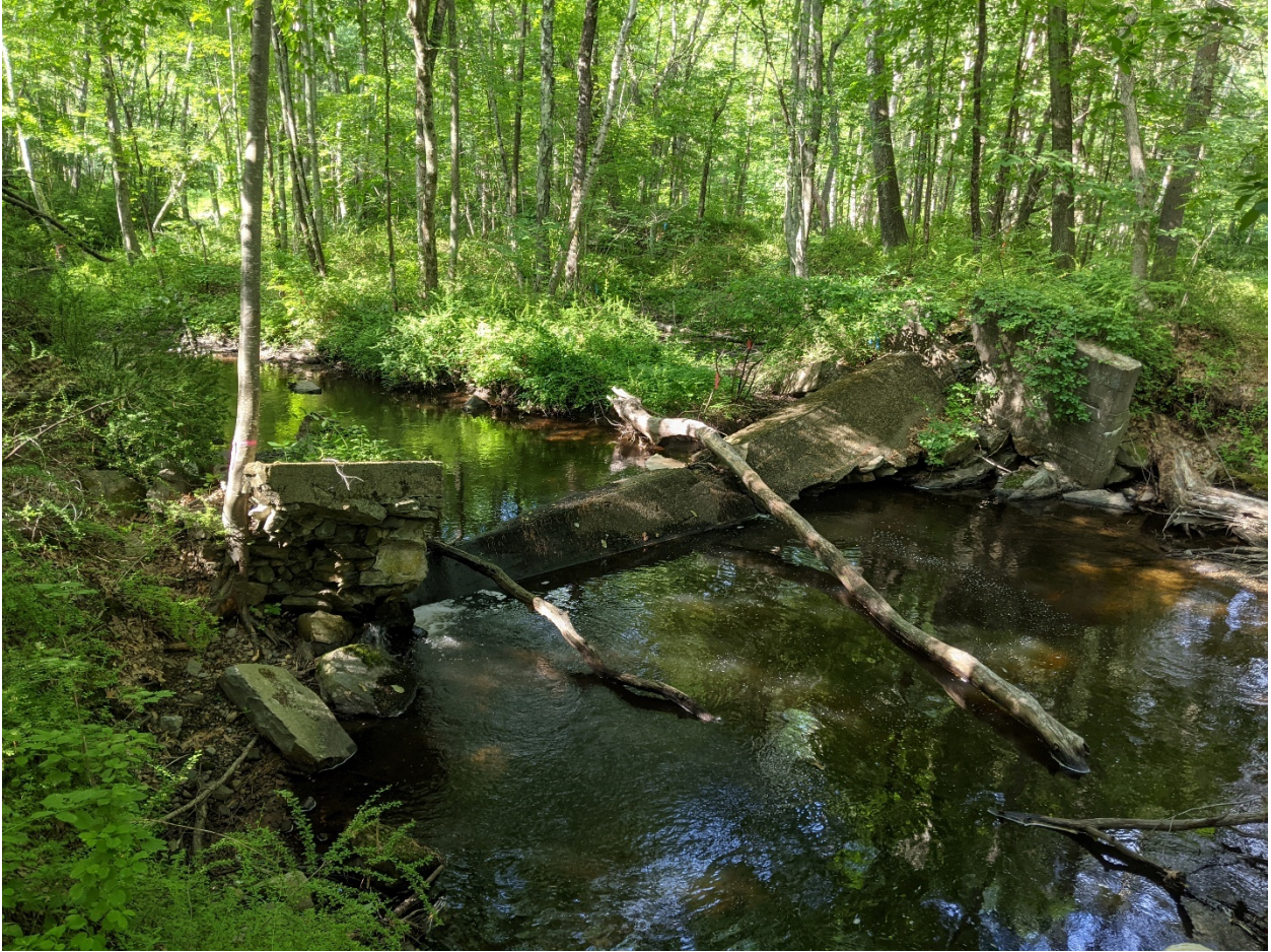
Photo 1: Overview of collapsed spillway from right embankment. Note water is flowing underneath the collapsed spillway on the left side.
